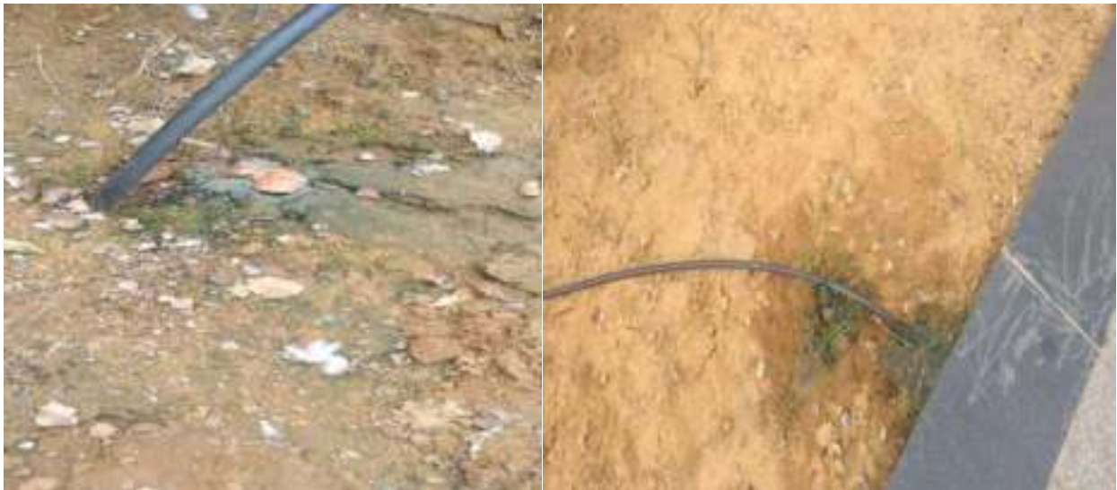
Figure 9: Images of water wastage around the facility
