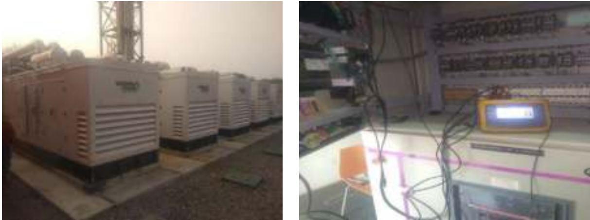
Figure 13: DG Performance Test
