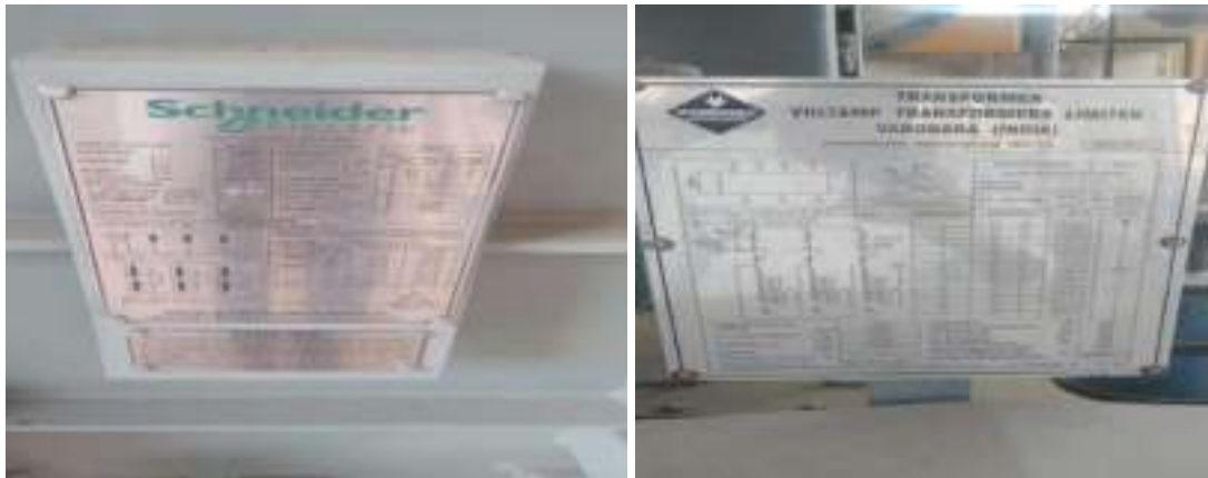
Figure 6: Name Plate details Transformers Installed at New Door
