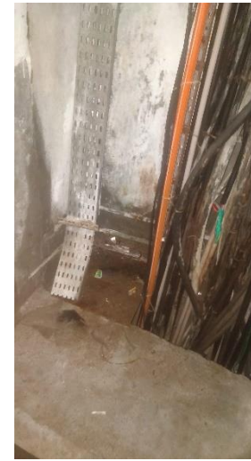
Image 7: Leakages in AHU rooms
