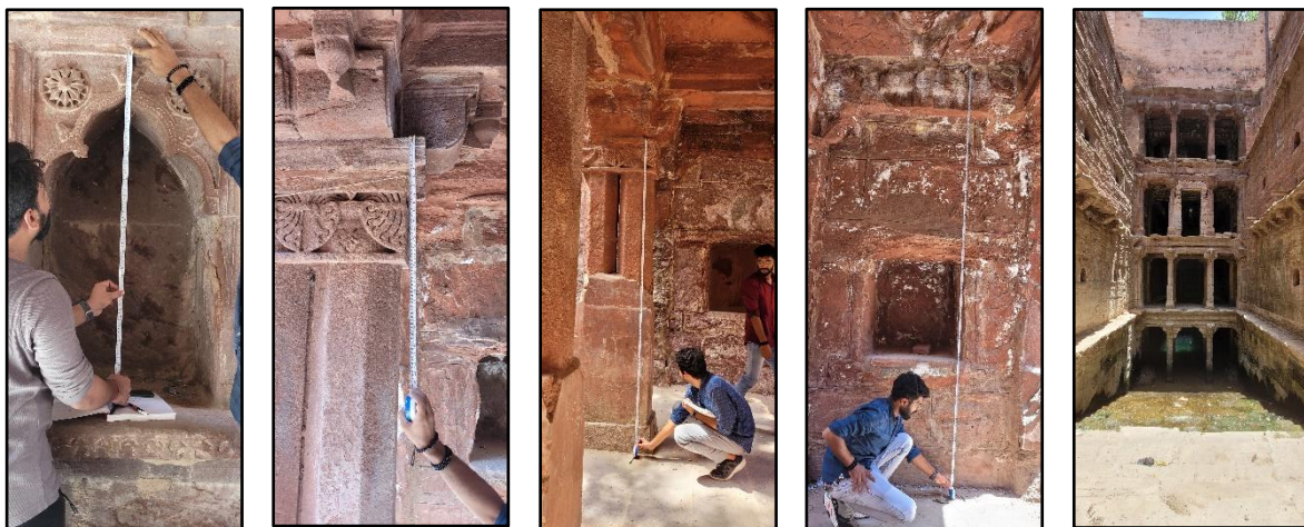
Photograph 1: Expert Team Visit to the Site "Tapi Bawari, Jodhpur"; Team getting the photographs for the preparation of the measurement drawing and condition mapping of the "Tapi Bawari, Jodhpur"
